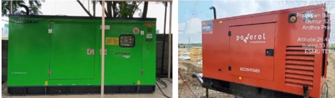
Figure 37: Acoustic enclosed DG sets to curve down the noise level
