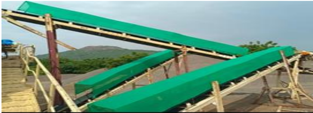
Figure 5-3: Green-nets covered conveyor belts, air quality monitoring and electric busses used for workmen transportation
