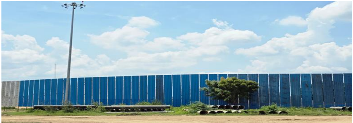
Figure 5-5: 7 meters height Barricades provided at the stock yard as Air Pollution control measure at BSR
