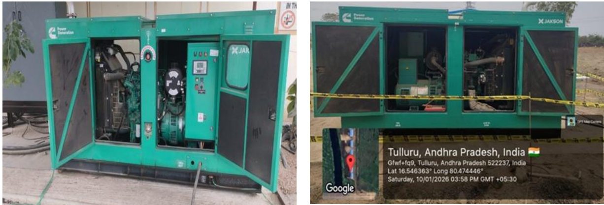
Figure 5-4: Acoustic enclosed DG sets
