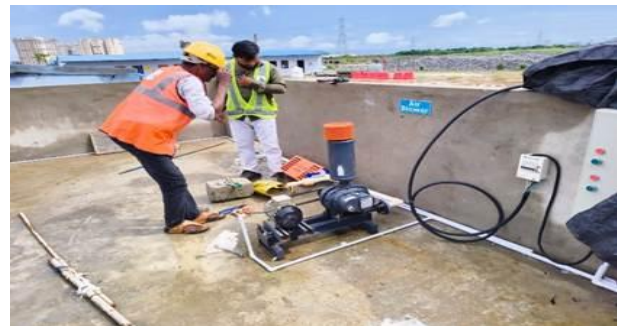
STP Air Blower
