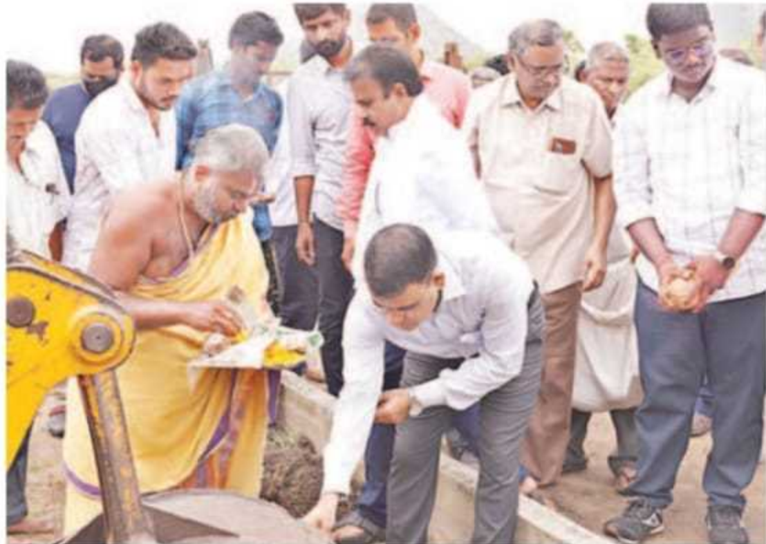
AP CRDA Commissioner Vivek Yadav laying foundation for development works at Pichikalapalem on Monday
